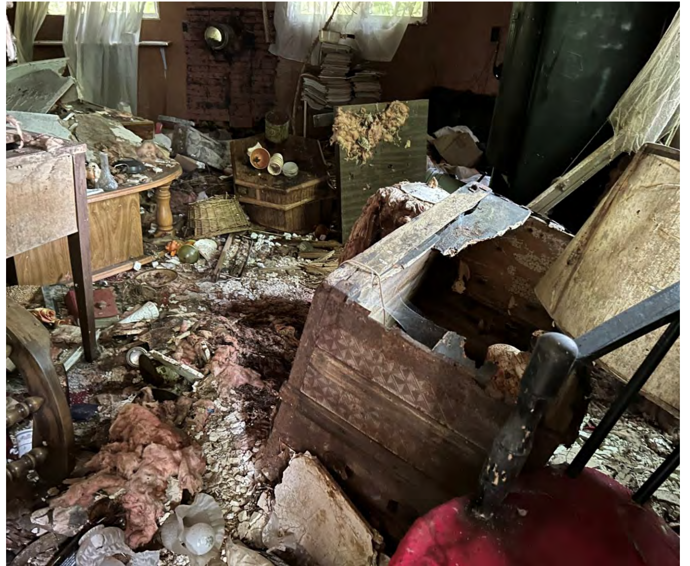
The buildings were a drug and drinking den and became a fire and safety hazard to the neighborhood.
