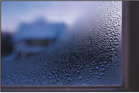
Condensation on the inside of a window-pane.
